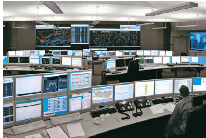
Fig. 7.2-14: View into a large power control center
