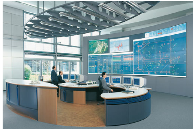
Fig. 7.2-5: Typical control room environment
